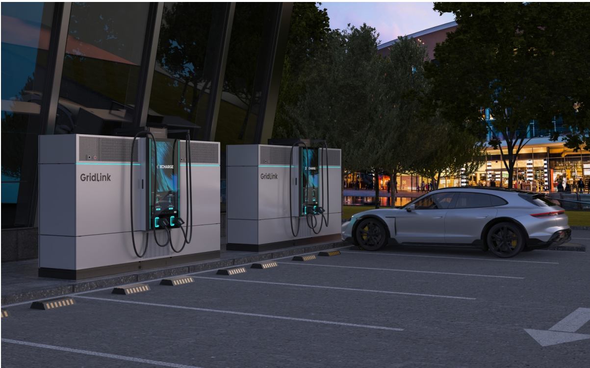
XCharge's GridLink chargers. Source: XCharge North America.
